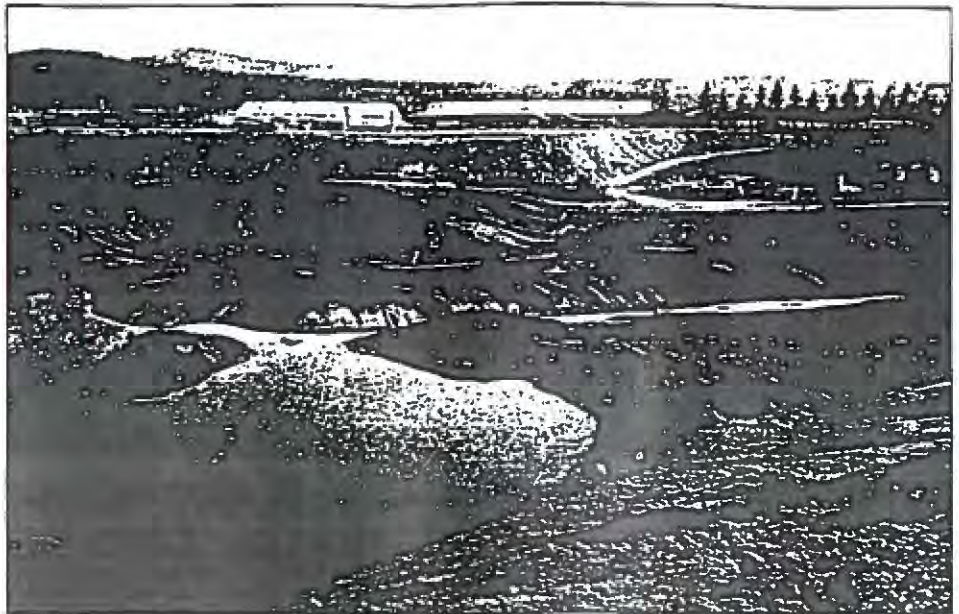
Figure 2. Moving earth and shaping the mined surface are important steps in reclamation. Shown is the Central Pre-Mix Yardley pit, where the central part of the pit is being shaped with gentle contours, canals, and islands. Subsequent uses of this pit are a heavy industrial area (concrete products) and a lake and wetland area for wildlife. (Photo by Mark Murphy, Central Pre-Mix)
