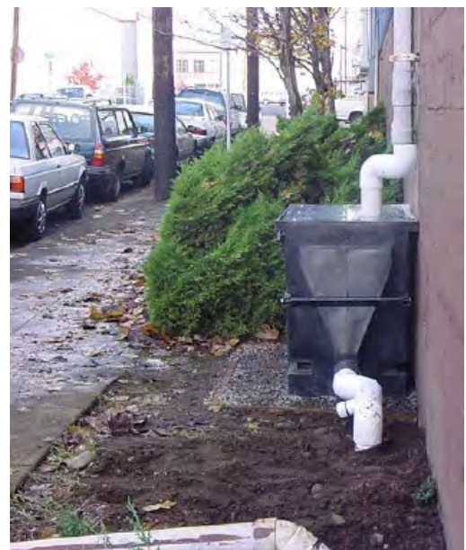
Roof Downspout type filter
