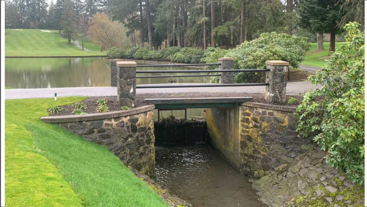
View east at water control gate that impounds Woods Creek and detains water for irrigation pond. View of downgradient side of water control gate.
