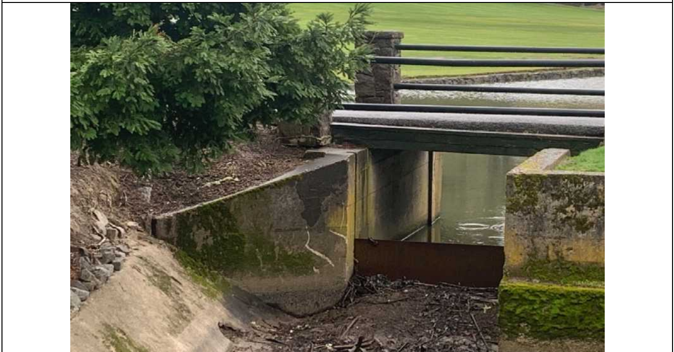
View southeast at water control gate between irrigation pond and Fanno Creek. View of downgradient side of water control gate. Floating debris from Fanno Creek is stopped from entering irrigation pond.
